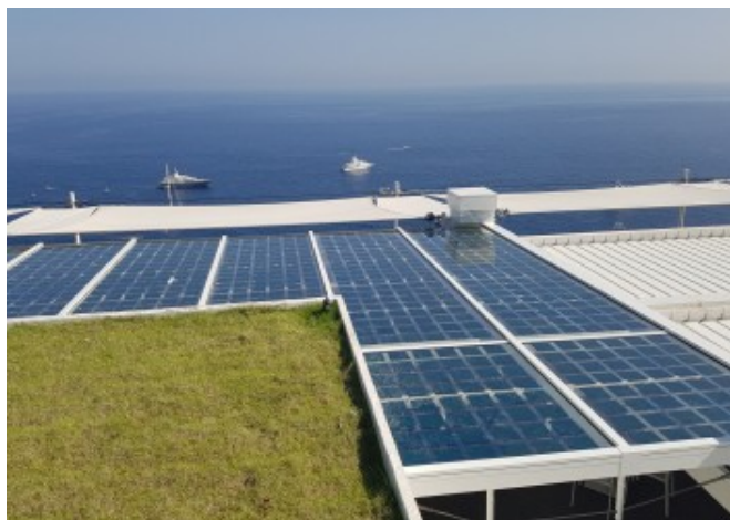
Close-up of a BIPV canopy © GruppoSTG Srl
