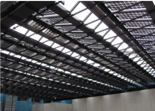
Detailed view of the BIPV plant bearing structure © Colterenzio Winery
