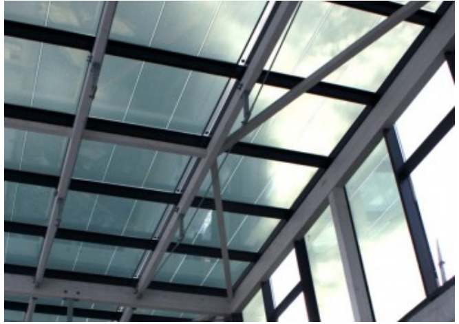
BIPV roof and façade on the entrance atrium © Onyx Solar
