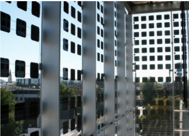
BIPV façade from the inside © Dieter Moor, ertex solartechnik GmbH
