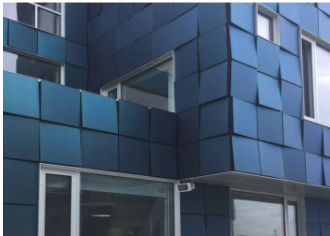
Detail of BIPV façade © Karin Kappel
