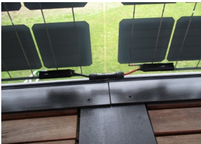
Detailed view of the modules cables junction © building owner
