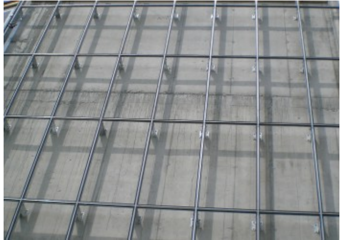
Steel system supporting the modules that cover the opaque building façades © Günther Wallnöfer
