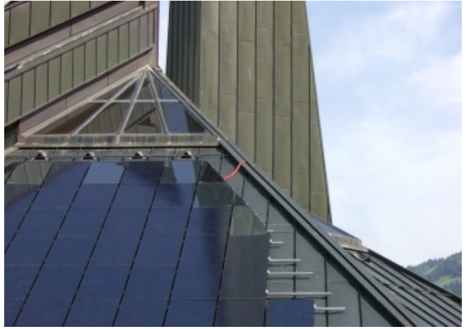
Construction phase, the church metal roof and the BIPV mounting system are still visible © Eurac Research
