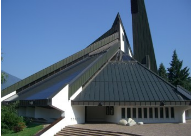
View of the original metal roofing surface, not so different from the PV modules © Eurac Research
