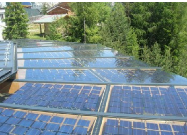
View from above of the BIPV glass roof: the visible ducts protect the electric connections © Augustin Clement
