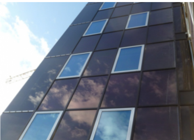
Enzian Office BIPV system: the modules replace opaque parts of the façade (under the windows high) and semi-transparent sections (beside the windows) © Eurac Research
