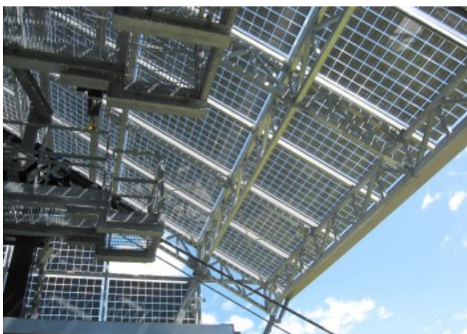
Steel trusses system supporting the BIPV plant © Leitner Electro Srl
