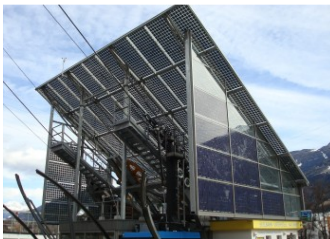
The ropeway station roofs were optimally tilted (30°) for the photovoltaic integration © Eurac Research
