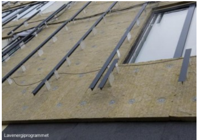
Black mounting brackets and modules give the façade a uniform appearance © Lavenergiprogrammet
