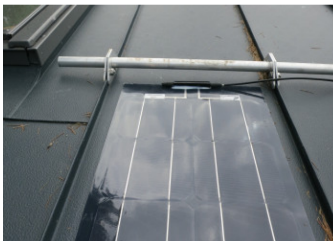
Detail eines Solbian-Photovoltaikmoduls © Myriam Perna, Arch. Valentina Cari
