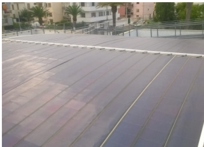
BIPV system on the roof © Alberto Ferrero
