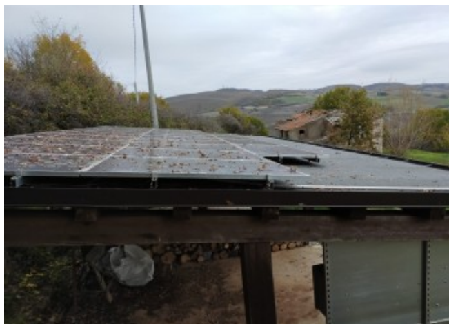
Detail of the mounting system for the photovoltaic modules © Arch. Patrizia Trivisonno
