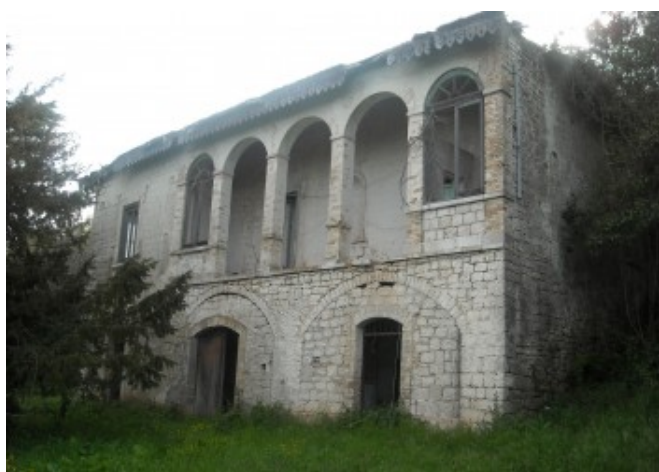
State of conservation of the south-south-east façade before the intervention © Arch. Patrizia Trivisonno
